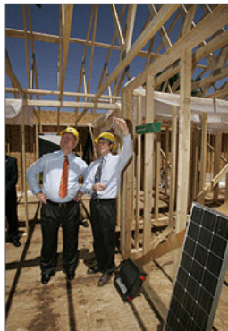
Secretary of Energy Samuel Bodman toured the construction of the home in 2005 with NREL researcher Paul Torcellini.
